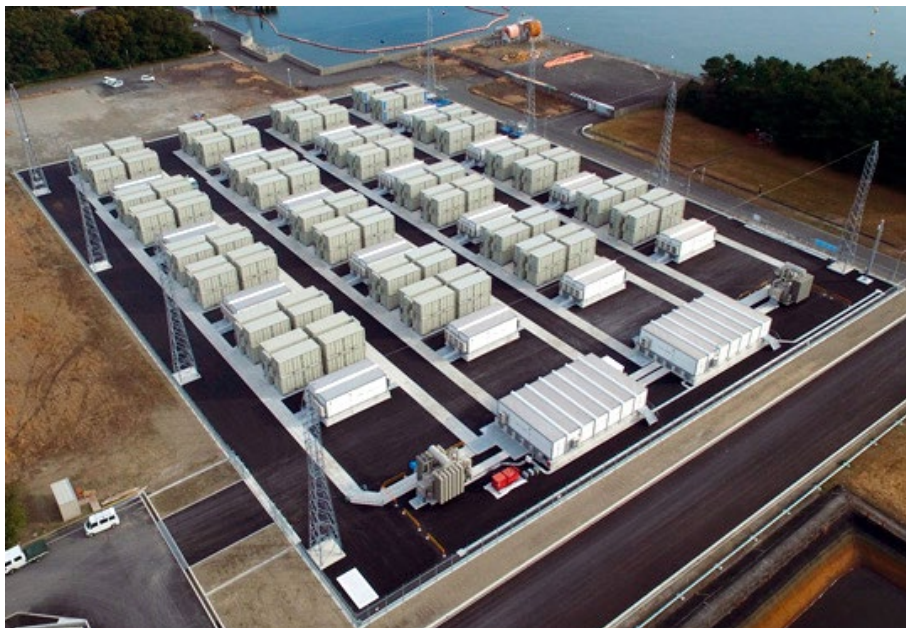
2 pav. Na-S baterijų saugykla Buzen mieste, Fukuoka (Japonija). Šaltinis: MITSUBISHI ELECTRIC News Releases Mitsubishi Electric Delivers High-capacity Energy-storage System to Kyushu Electric Power's Buzen Substation.
