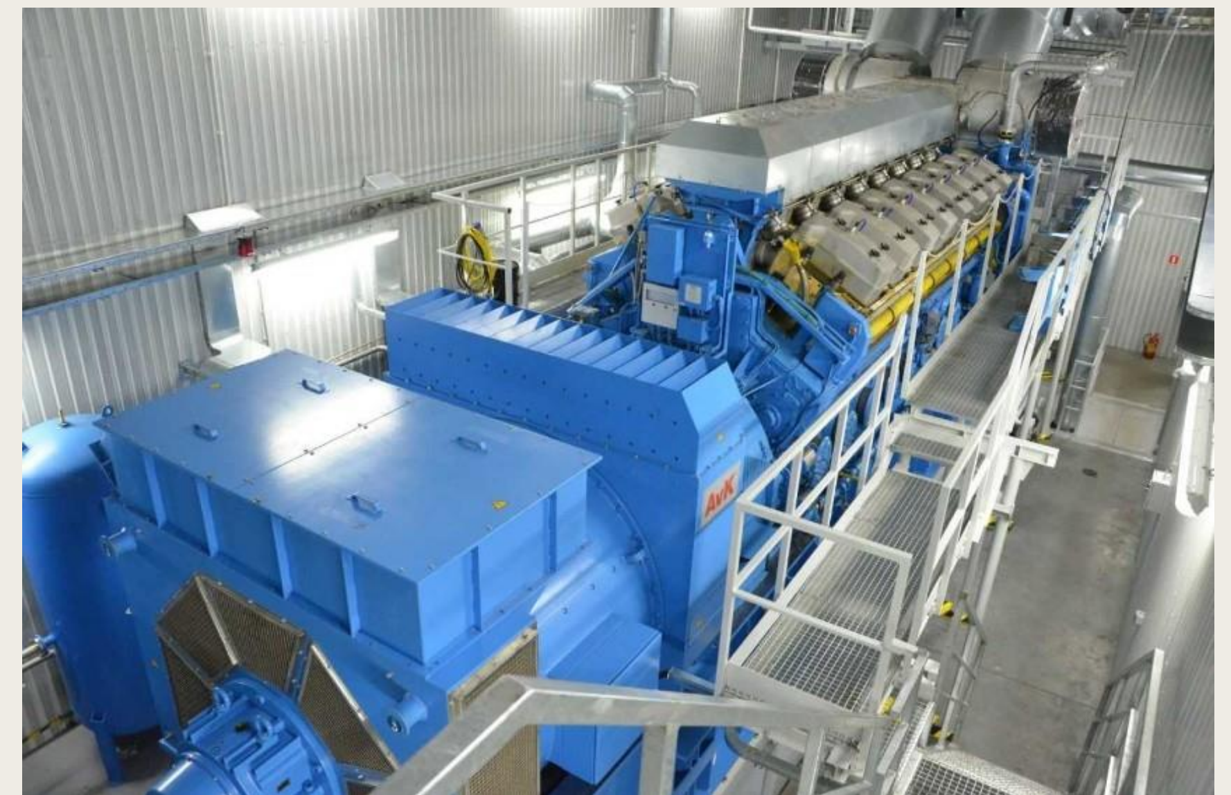
Cogeneration Rolls-Royce engine in Wejherowo
