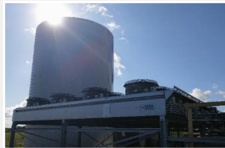
To add flexibility to the heat production and create balance between supply and demand, a PTES can be integrated with the existing energy infrastructure eg. an integrated heat pump system or an integrated system consisting of a solar heating plant and a heat pump
