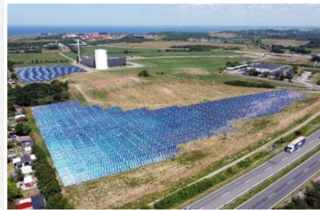
By integrating a PTES with a solar heating plant, excess heat produced during summer can be stored and released during winter, when the heat and hot water demand increases.
