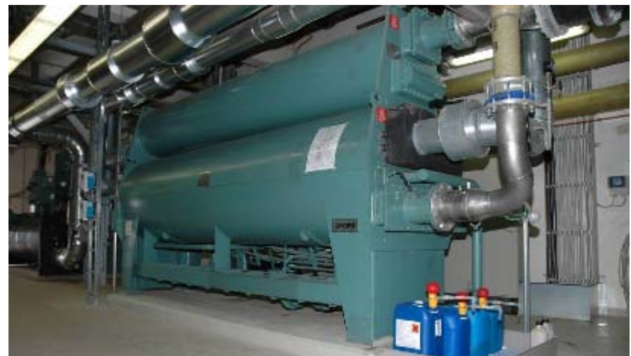
Absorption chiller unit 500 kW
