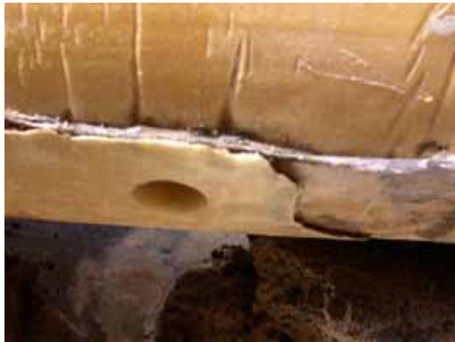
Figure 8. Crumpled polyethylene foil. Defect in the PUR foam from the production process.
