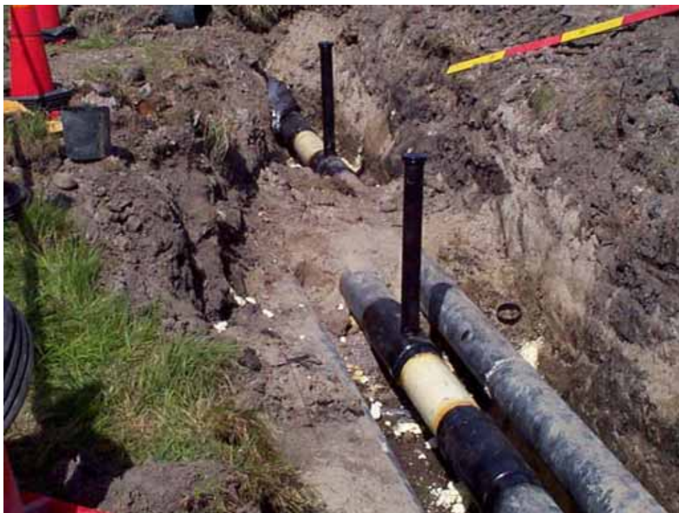
Figure 1. Installation of casing free pipes in Hisings-Backa, Sweden. North direction is towards the top of the photograph.
