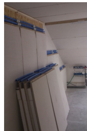
Fig. 4. Heat storage modules
