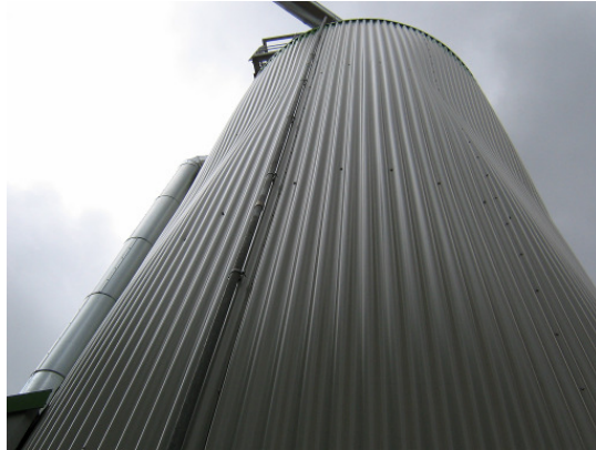
Damaged hygienisation tank cause depression
