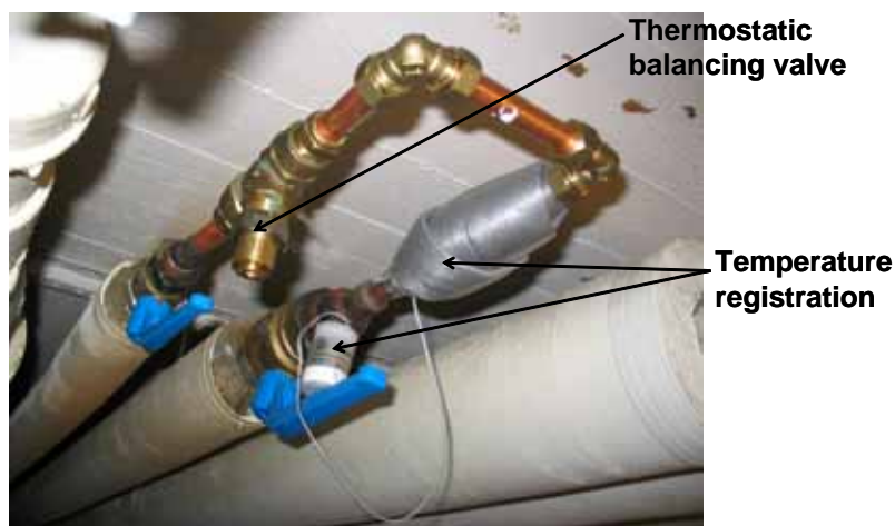
Figure 3 Thermostatic balancing valve installed at the end point of DHW circuit
